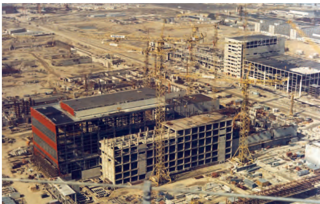
VÝSTAVBA BUDOV STROJOVNY A ROZVODNY CONSTRUCTION OF THE BUILDING OF THE MACHINE ROOM AND THE BUILDING OF THE SWITCHING STATION
