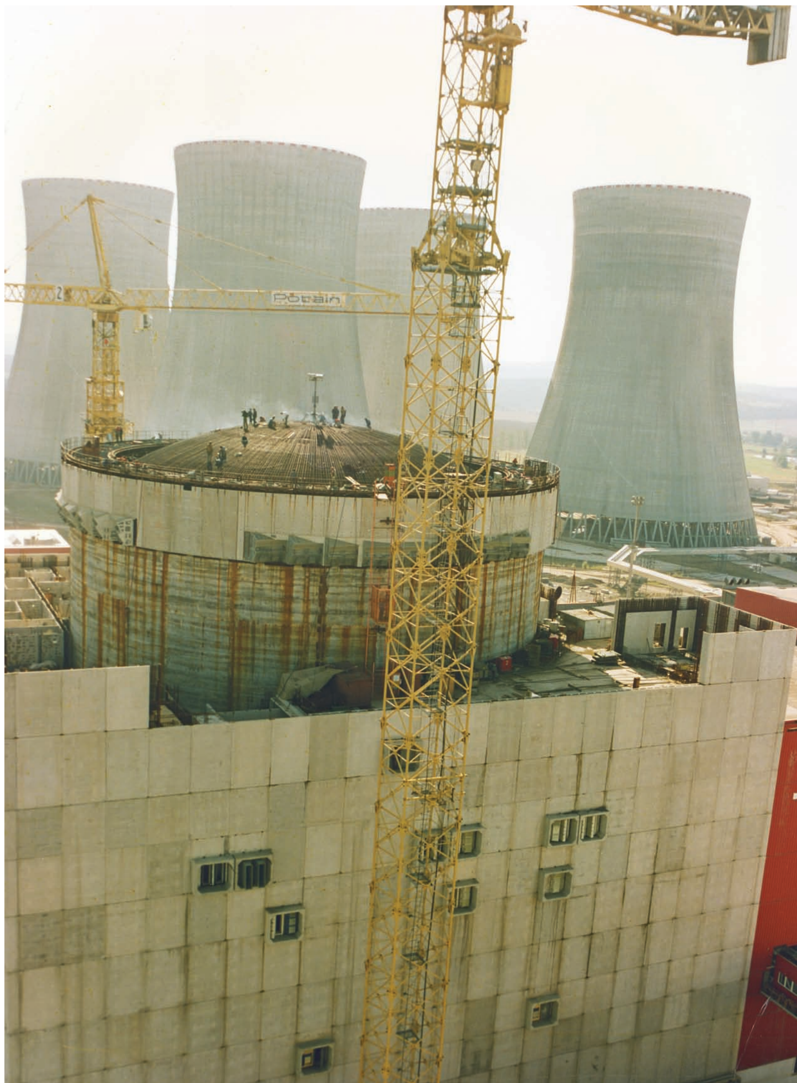
PRÁCE NA OCHRANNÉ KOPULI BUDOVY REAKTORU | WORKS ON THE PROTECTIVE CAP OF THE REACTOR BUILDING
